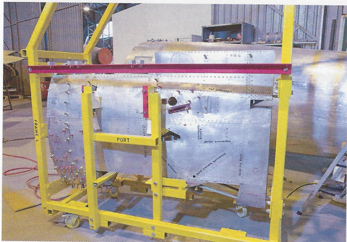
The custom-built jig around the original tail section. Note where the team has marked up the skins to show the various rib identities and locations.
